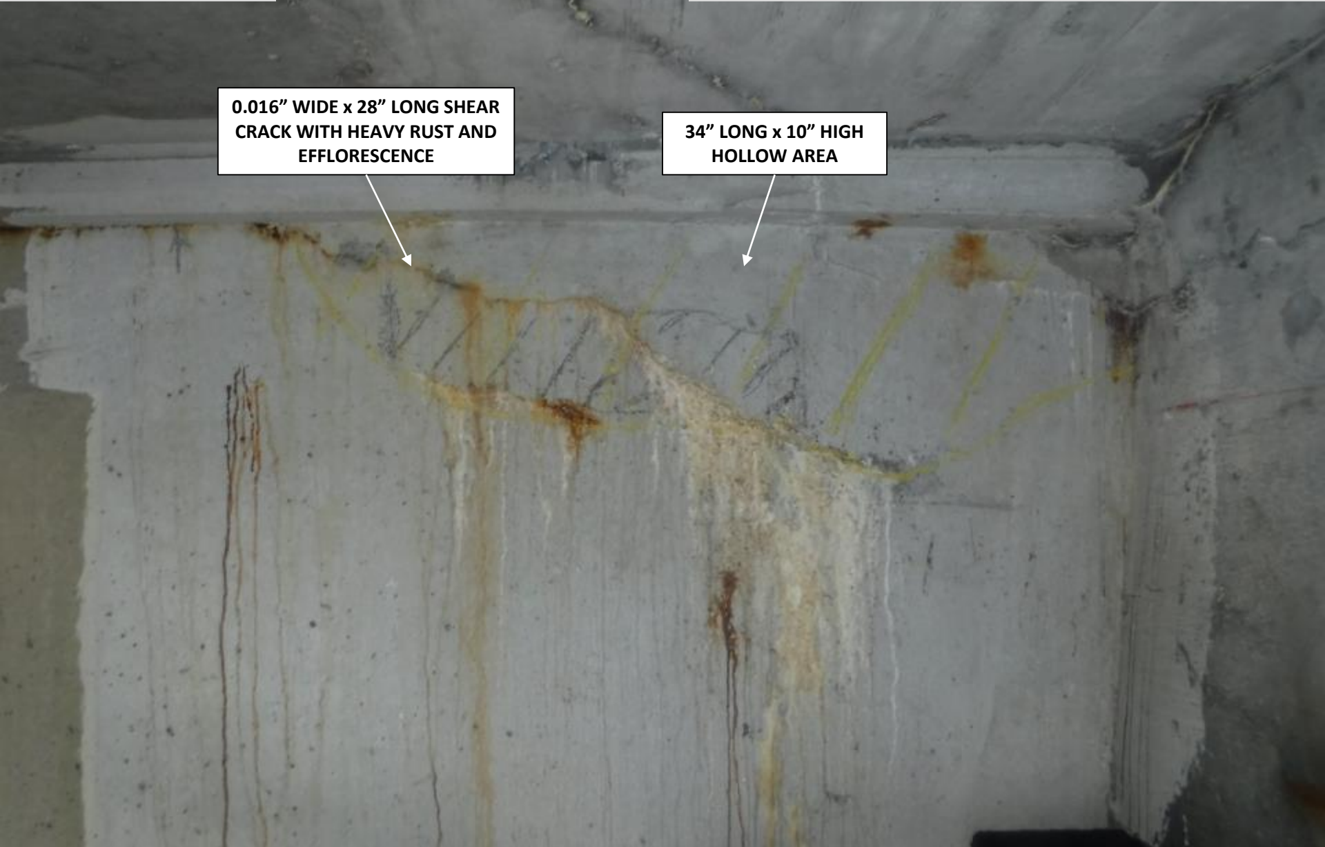
DROP-IN GIRDER 'F' – NORTH FACE AT WEST CORBEL IN SPAN #3 (LOOKING SOUTH)
